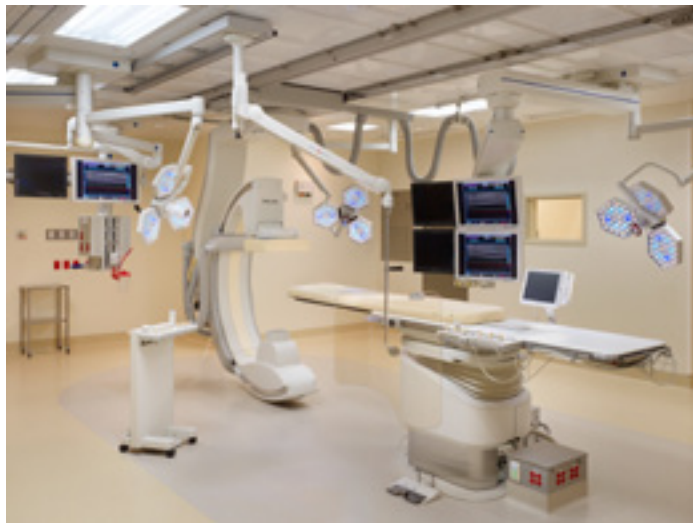
Unistrut in Hybrid Operating Room - Photo Courtesy of Bruce T. Martin © 2011
